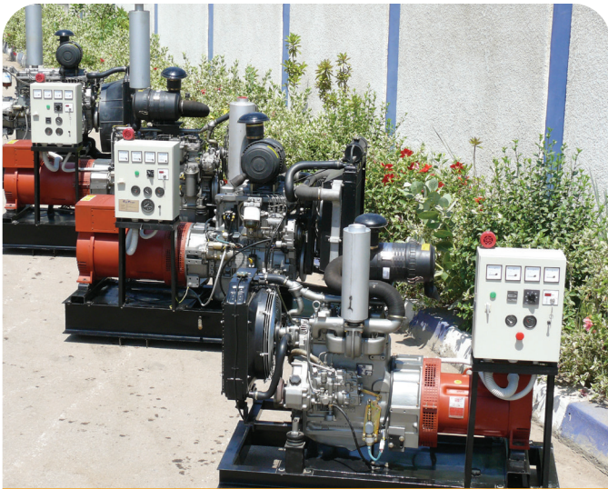
Open Diesel Generators
